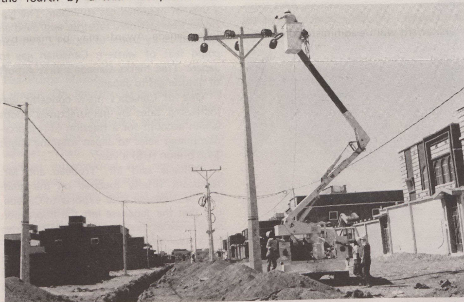
This distribution pole, mounted in a central Saudi Arabian town, is part of a major electrification program in the El Qaseem region, for which Canada's SNC Group is providing engineering, procurement and construction management services. Some 6 800 kilometres of distribution line and 965 kilometres of transmission lines are being built.
