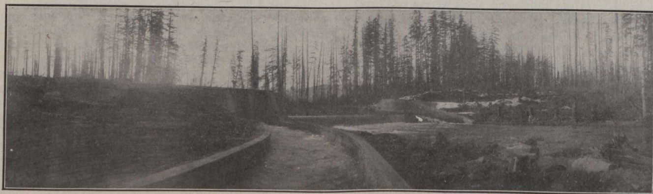
Diversion Dam with Beginning of Masonry-lined Canal. Note Fish Ladder on Right.
