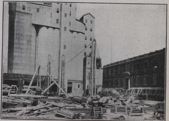
Fig. 3.—Operations Commencing on the Construction of the Second Addition to the Commissioners' Elevator No. 1.
