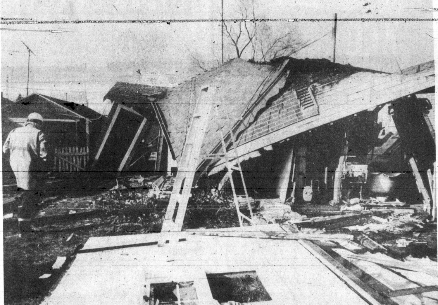
An official of Ontario fire marshal's office moves in to inspect remains of a Ninth Street home in Lakeview which was rocked by explosion Thursday. No cause has been determined in blast which blew out two walls and seriously injured one man. (Times photo by Ray Saiz)
