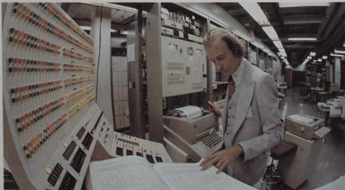
The switching system developed by Bell Northern Research for Northern Telecom.
