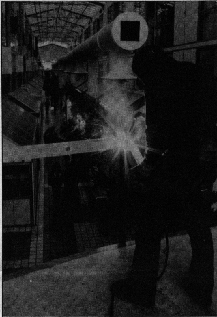
Yes there really will be new lounge space in HUB mall as promised. Patrick Beacon, Delmar Steel employee, works on a structural expansion of a lounge at HUB's south end.
