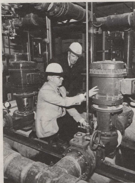
Al Hendry (front) and John Doull examine the pump of the cooling system installed in Halifax, Nova Scotia's new commercial complex, Purdy's Wharf.
