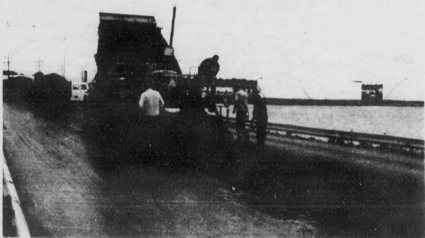
Ice Free pavement courtesy The civil department
