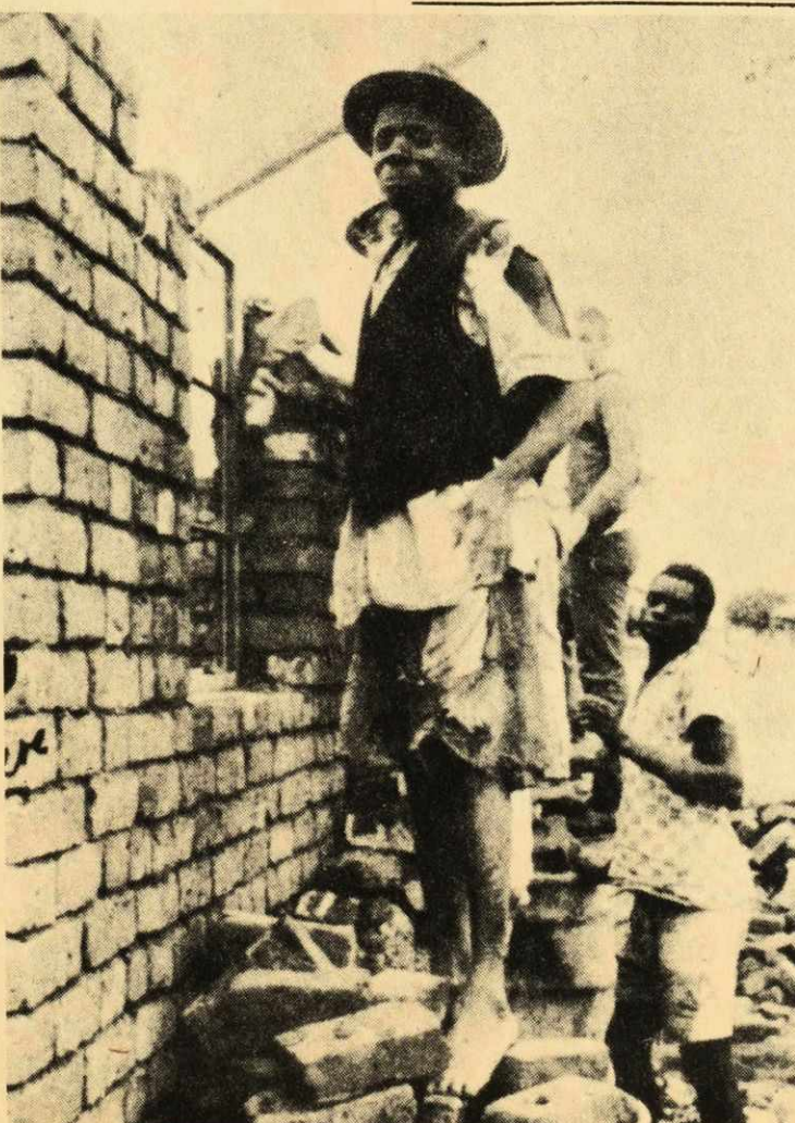
Bill Curry hard at work building a house which is to be part of the St. Francis Hospital complex.
