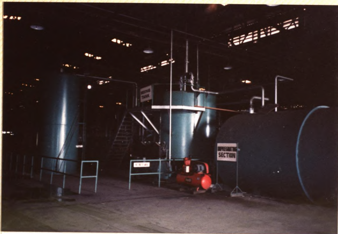
No. 20. Solution tanks in wood preservation section.
