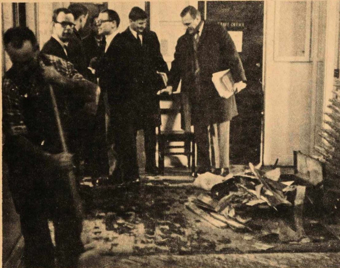
The workman is repairing the floor in the Arts Annex. Steam fittings broke below the wood timbers, causing them to swell and rise. Does this mark the beginning of the end for our beloved Arts Annex... only the Administration knows for sure.
