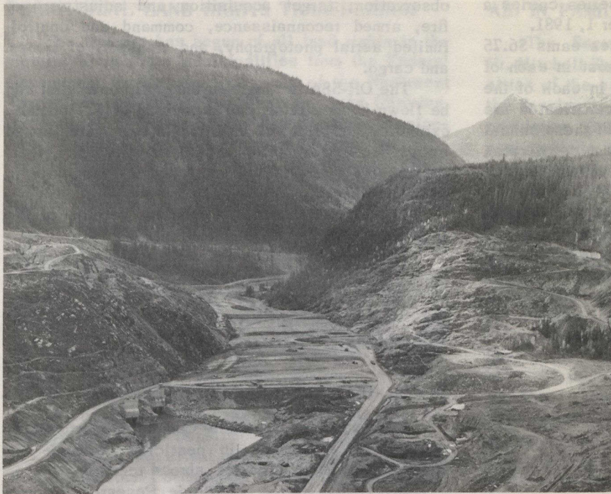
The aerial photo of the Mica damsite, near Revelstoke, B.C., looking downstream, shows intakes for the diversion tunnels (near bottom left of picture).
