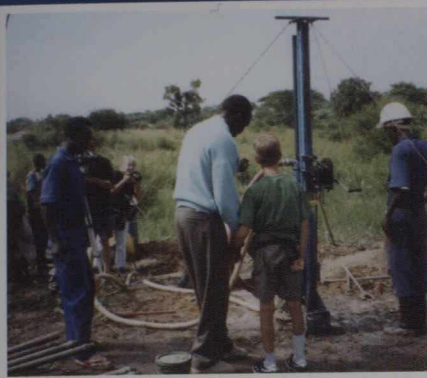
Ryan watches the drilling of the first "Ryan's Well" in Uganda. He has helped to contribute funds for wells in Ethiopia, Malawi and Zimbabwe, and is working with Canadian Olympic gold medal wrestler, Daniel Igali, to build a well and school in Nigeria, Daniel's birthplace.
