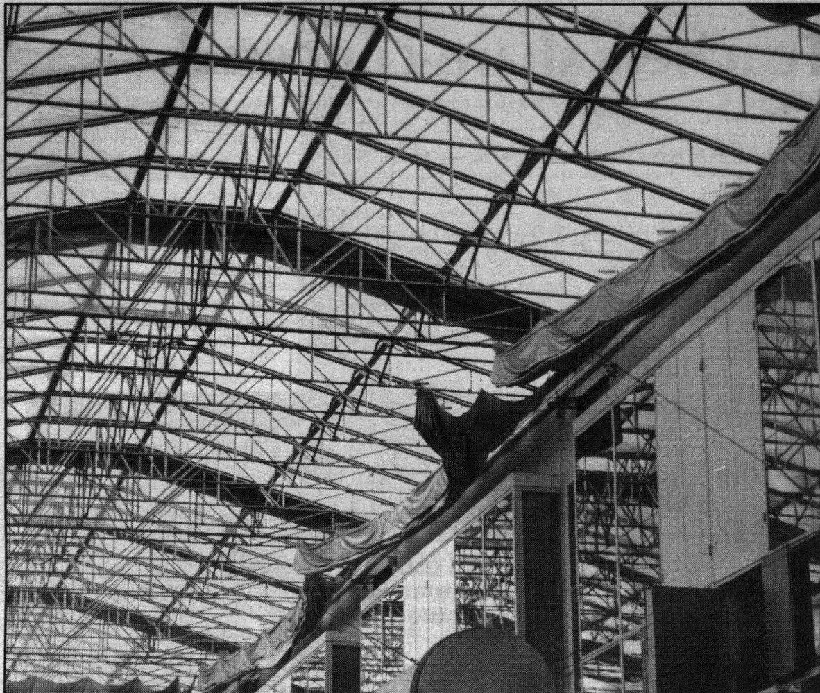
Until the university repairs HUB roof, carry an umbrella
