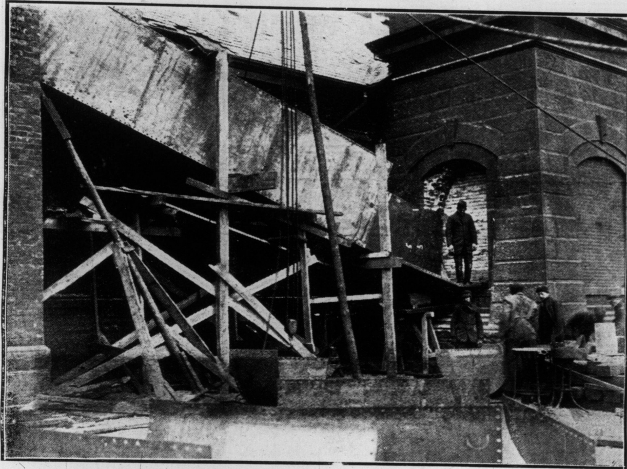
KEEPING ABREAST WITH THE TIMES. City employes putting in a smoke consumer at John-street water works station.
