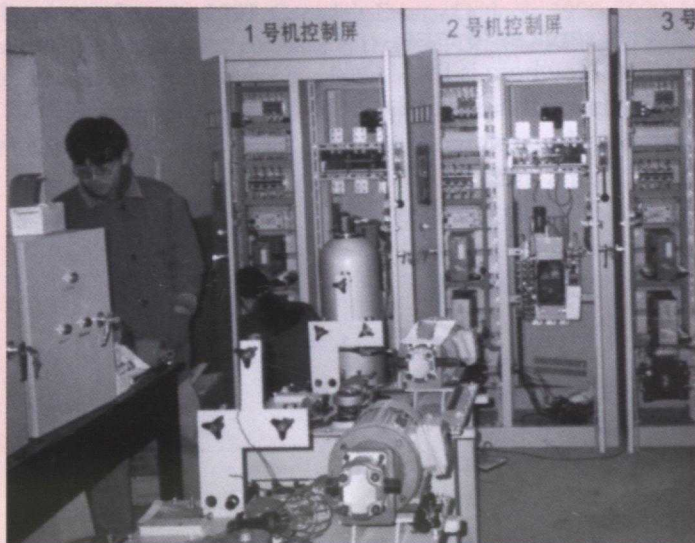
Small hydro automated control unit in China.
