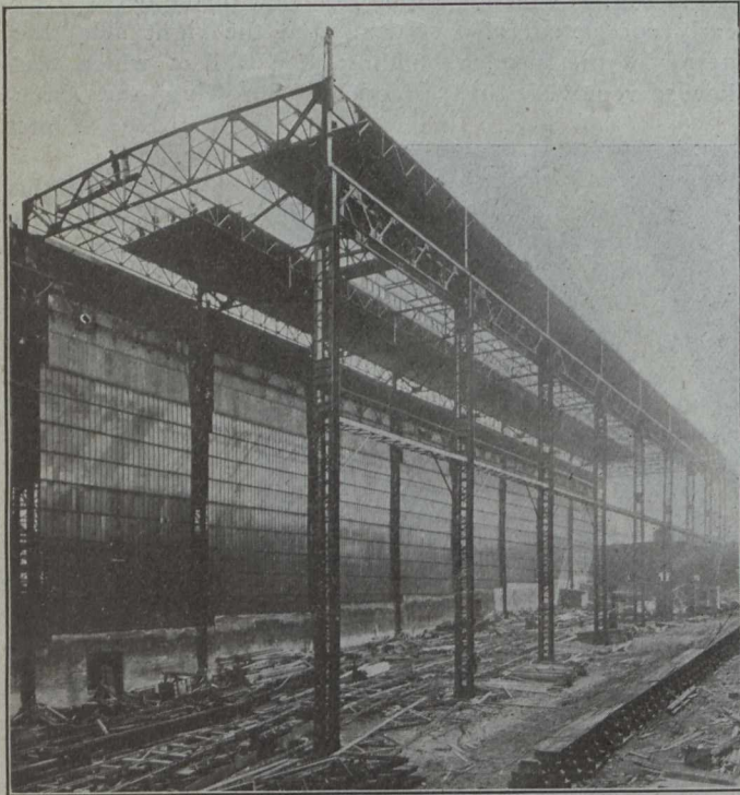
Fig. 2.—Erection of First Section of Berth. All the Glass and Sash in the Side of Adjoining Building was Later Removed
